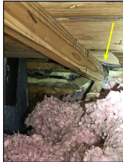
Stains around the chimney. I could not test this with a meter but the ceiling below was wet in the upstairs bathroom.
