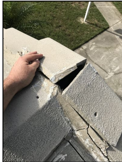
Loose rake tiles
