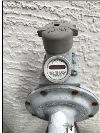
Tanks were empty. Could not test fireplace function because of this.
