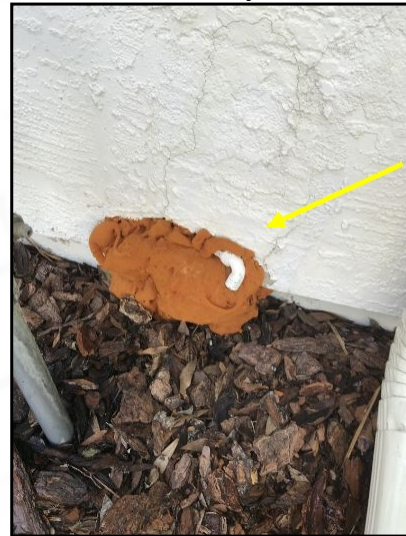
Unprofessional repair. Expanding foam will decay in sunlight. Recommend having a licensed professional repair this area
