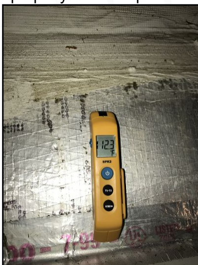
Heating temperature for the downstairs unit was 112.3 degrees.
