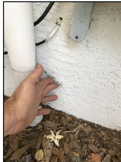
Ground wire has been cut off from the ground rod.
