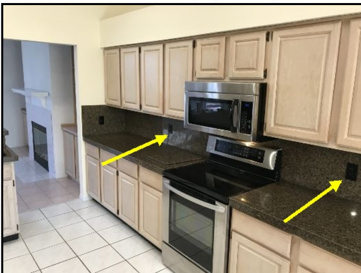
These outlets on the right side of the kitchen show an open ground. This should be corrected by a licensed electrician.
