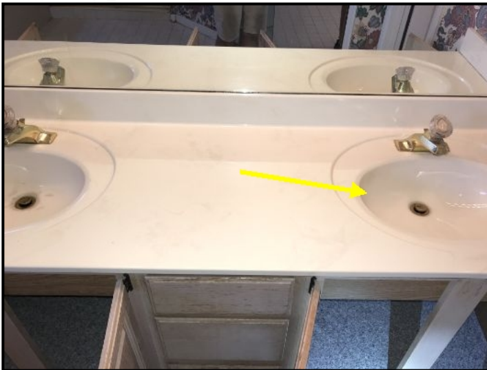
Sink on the right in the master bath is clogged
