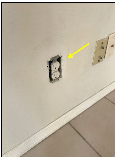
Missing cover plate in the living room
