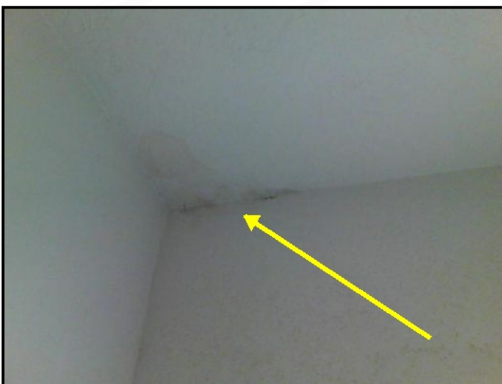
Stains on the ceiling in the upstairs bathroom
