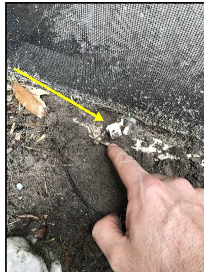
The pool enclosure is not connected to the bonding grid.
