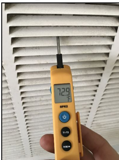
The return temperature for the test was 72.9 degrees. Both systems produced an adequate temperature differential in both cooling and heating modes indicating they were working properly at the inspection.
