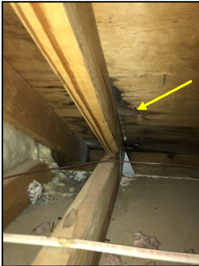
Active leak above the garage
