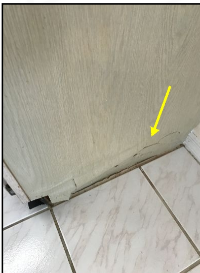
Damage to the cabinet
