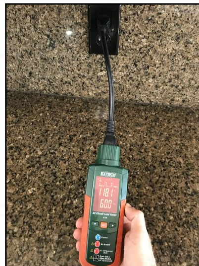
Tester showing open ground outlets
