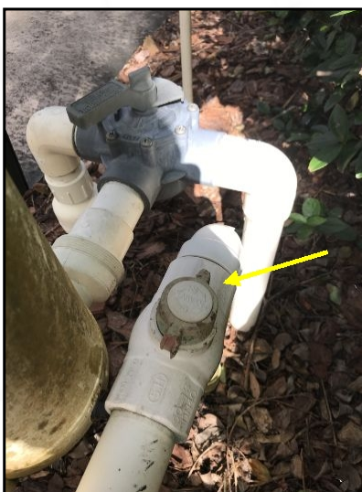
Broken control valve handle
