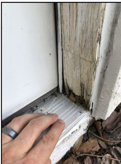
Wood decay around the exterior garage door
